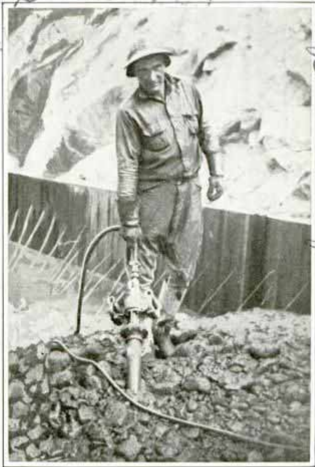
Vibrator for Making Concrete More Compact Is Shown in Operation; It Is Air-Powered
