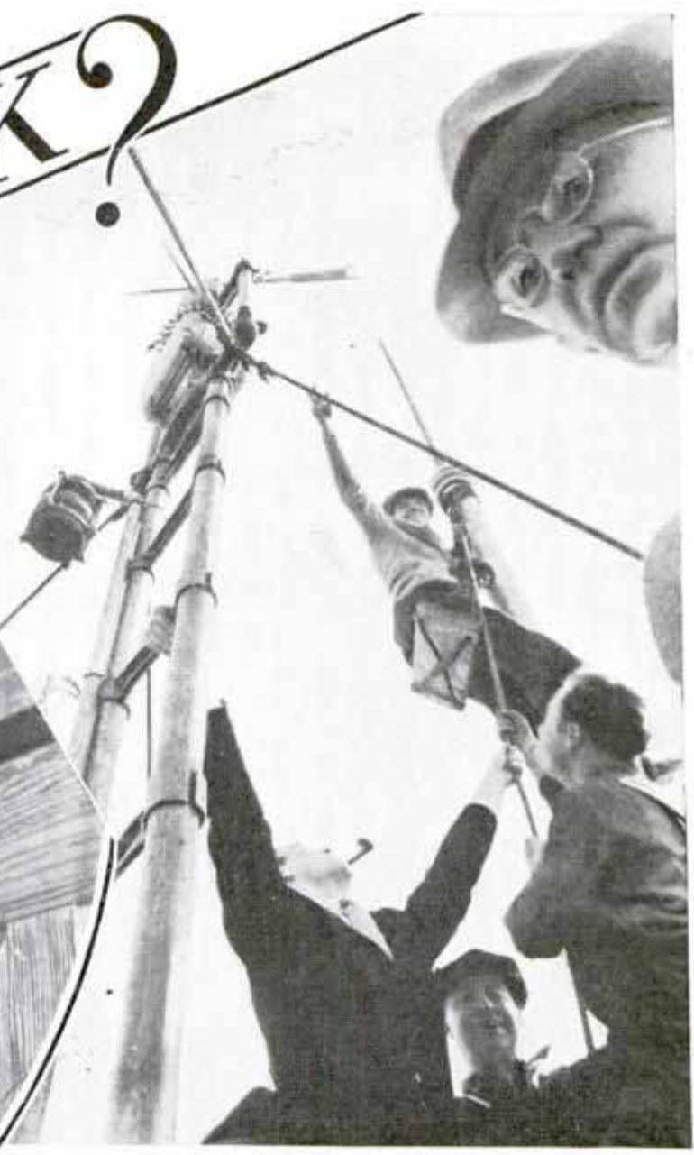
Above, Installing Lightning Arrester on Empire State Building to Protect Antennae of Experimental Television Apparatus
