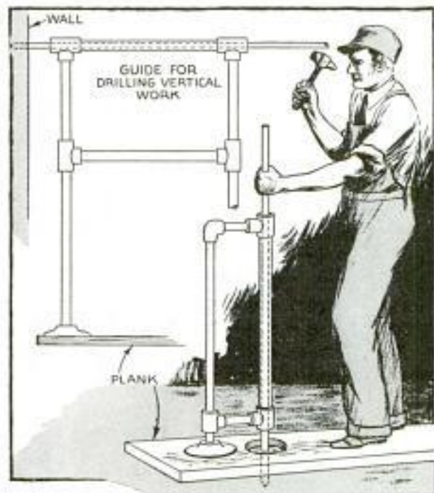
Two Guides That Help in Drilling Vertical and Horizontal Holes in Masonry with Star Drills
