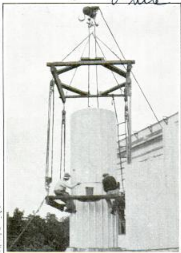
Swinging Scaffold Suspended from Derrick Which Saves Much Time and Labor in Setting Marble Columns
