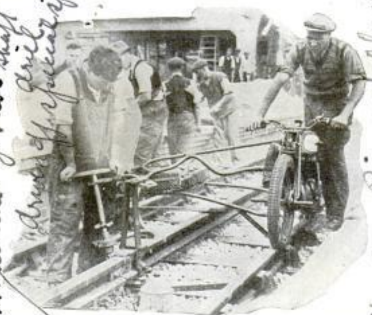
Power for Electric Drill Used in Railroad Construction Is Supplied by This Motorcycle Equipped to Operate on Track
