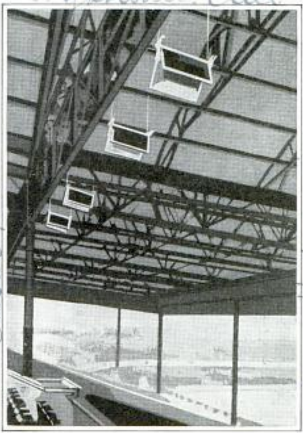
Electric Heaters Are Shown Suspended from Roof in Novel Method of Warming Grandstand
