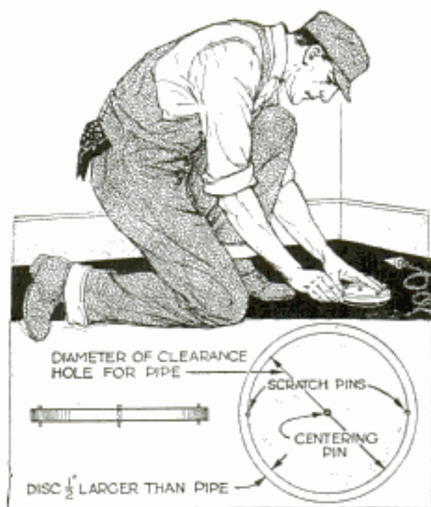
Marking Device and Plumb Bob Used to Lay Off Holes for Installing Vertical Pipe
