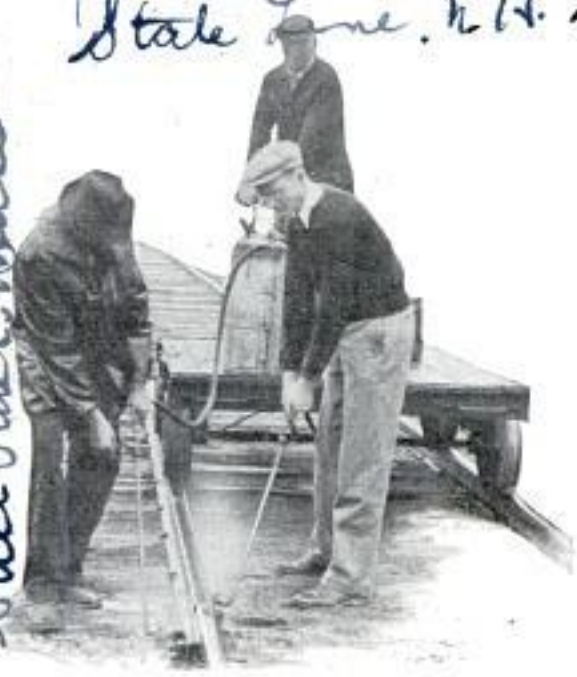
Replacing the Hand Method of Track Oiling, This Outfit on Hand Car Speeds Up the Job
