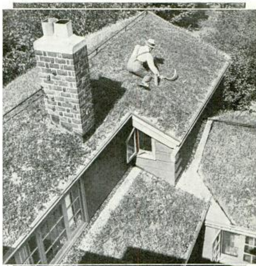
Comfort for Warm Weather Can Be Obtained by Planting Grass on a Roof; Note How It Can Be Trimmed During the Growing Season
