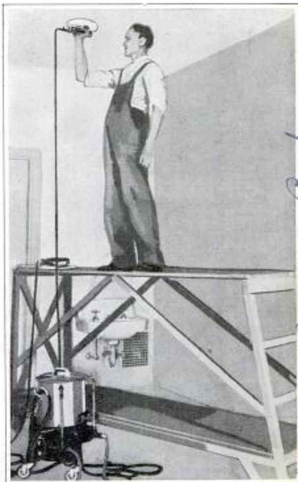
Using an Electric Washer to Clean Walls and Ceilings; the Machine Also Rinses the Surface
