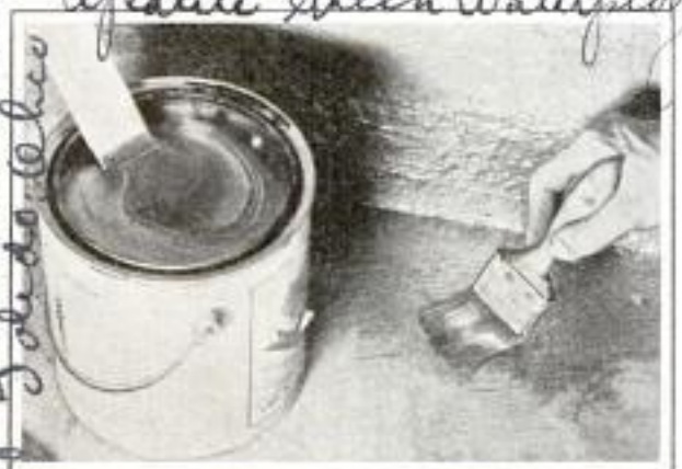
Covering a Concrete Floor with a Special Paint Which Seals the Surface against Moisture
