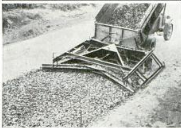
Rock Spreader Operated by Two Men; It Handles over 1,000 Tons of Material a Day
