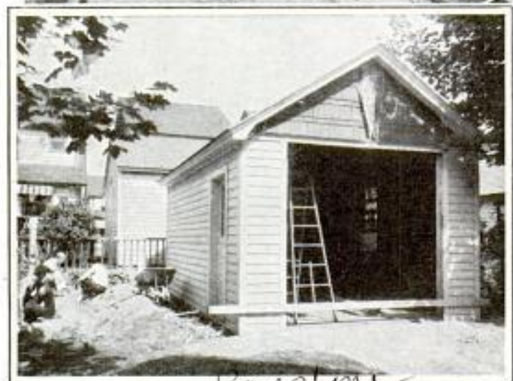
One-Car Garage Was Made to Accommodate Two Autos by Sawing It in Half and Extending Sides
