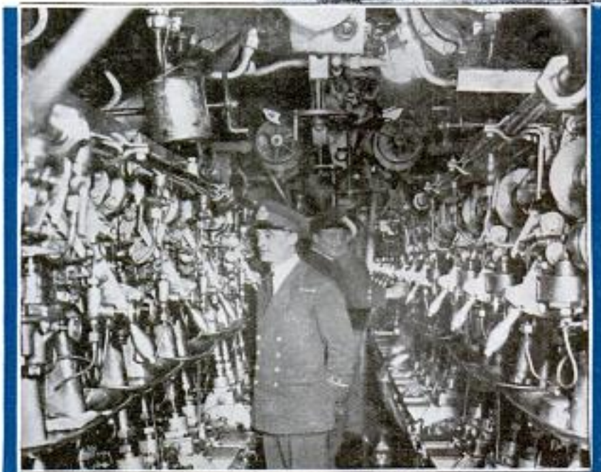
Photos © Kerstone Top, at the Periscope in the Control Room of a Submarine; Bottom, Engine Room of a Modern British Sub
