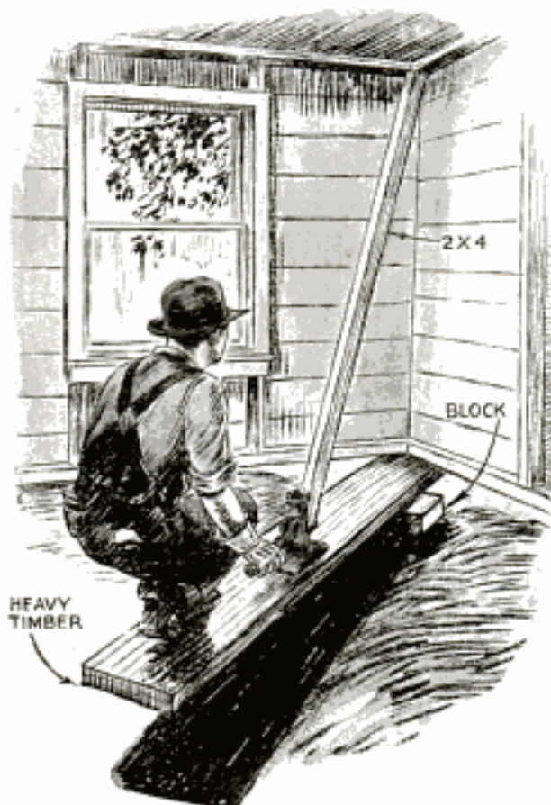
Corners of Small Buildings with Rotted Sills Raised with Jack Exerting Double Leverage
