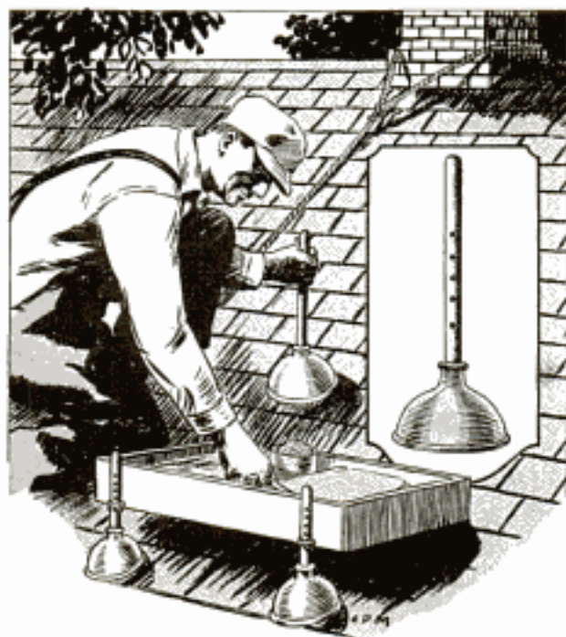
Rubber Sink Plungers Hold Toolbox and Steady Worker When Repairing Slate Roof
