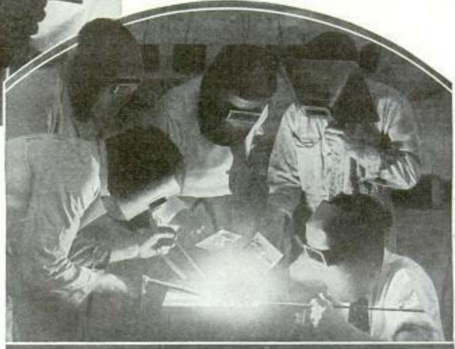
Top, Welder Holding the Arc Torch; Note Mask Which Is Worn to Avoid Sunburn Effects; Bottom, Several Torches Are Being Used on One Job
