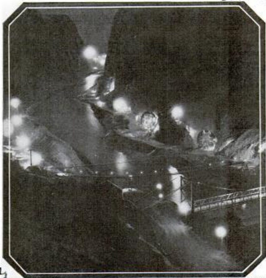
Canyon Where Hoover Dam Is Being Constructed Is Turned into a "White Way" at Night by Dishpan Reflectors behind Lights
