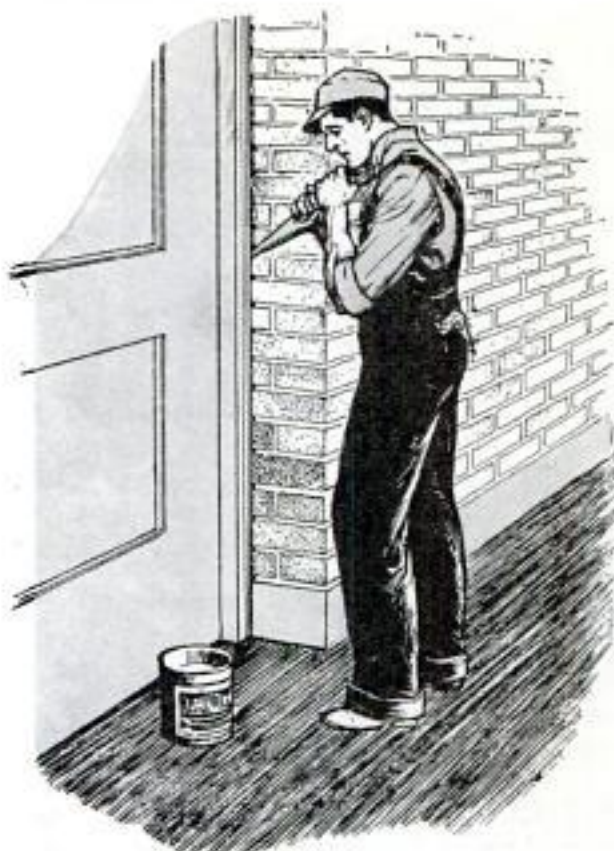
Calking Compound Forced into Cracks around Door with Gun Improvised from Paper Cone
