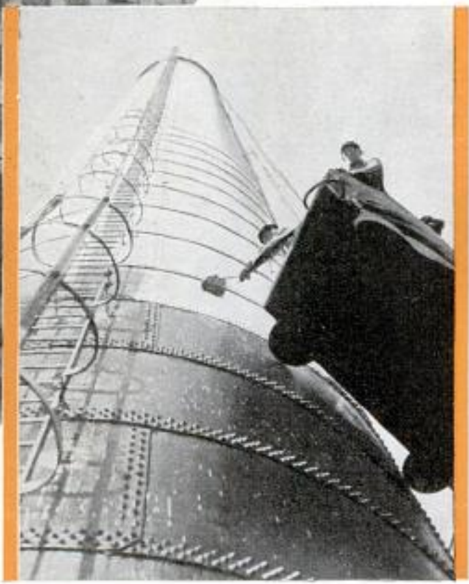
Top, Holding Aloft Two Ten-Foot Beams of Magnesium Alloy, Weighing Thirty Pounds Each; Above, Applying Aluminum Paint
