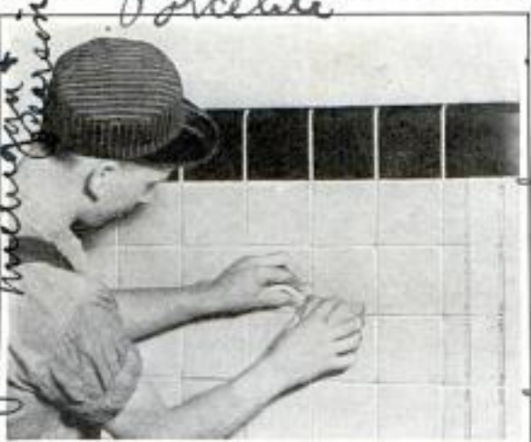
New Colored Steel Tile Is Clipped on a Backboard, Applied Directly to Wall
