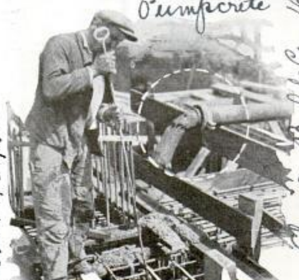
Pumping Concrete through Pipeline Direct to the Forms from Mixer 500 Feet Distant
