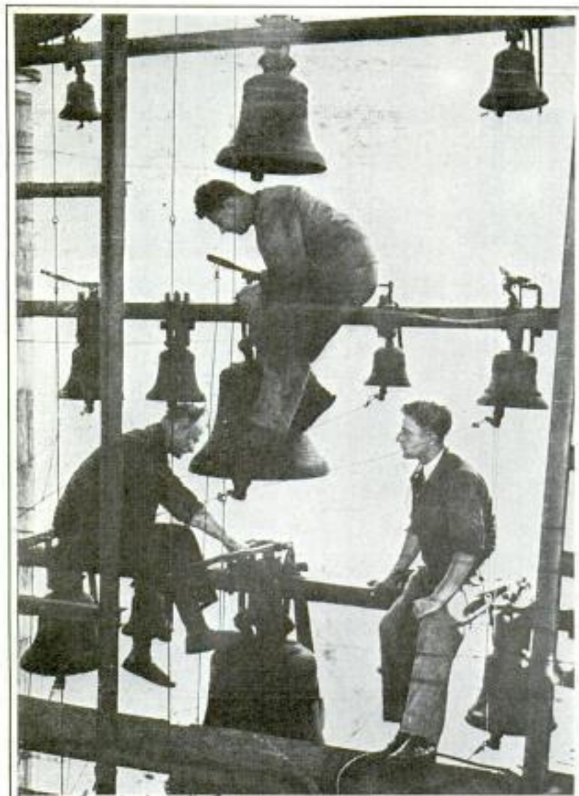
Wide World Workmen on Tower of the Potsdam Military Church Engaged in Repairing the Famous Chimes to Restore Tones of the Bells
