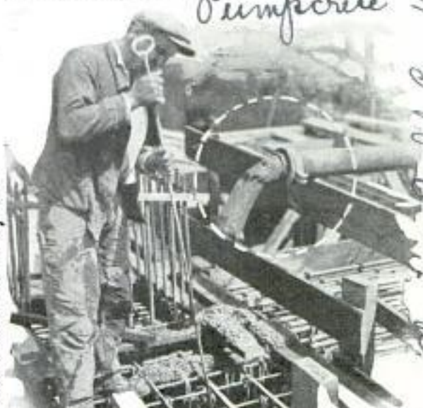
Pumping Concrete through Pipeline Direct to the Forms from Mixer 500 Feet Distant
