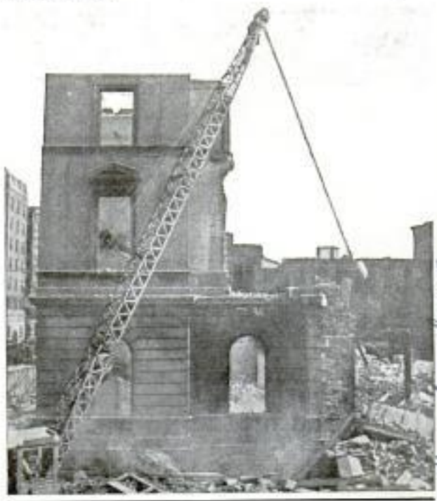
Battering Down the Stone Walls of a Building with Swinging Hammer Attached to Crane
