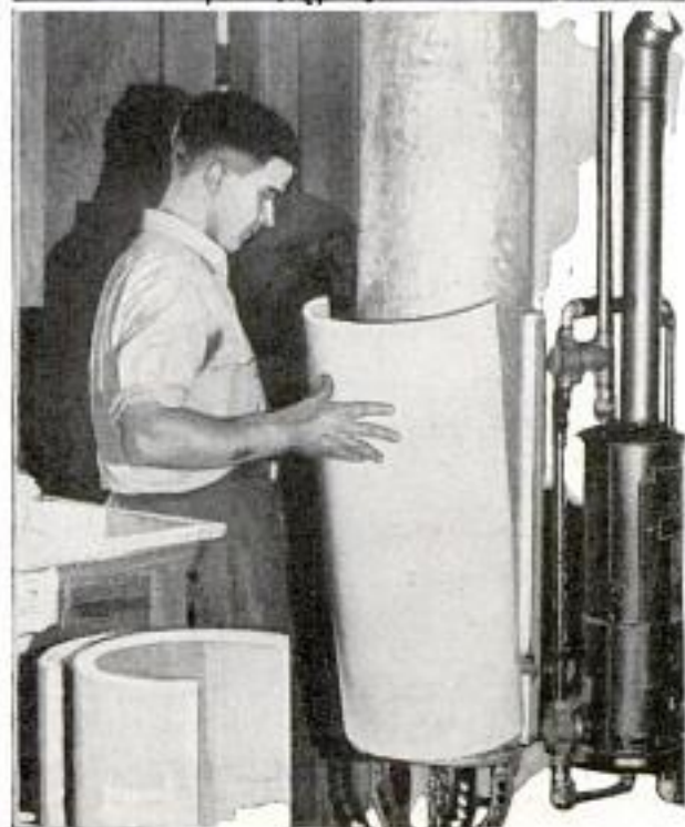
Installing Insulating Jacket around Hot-Water Tank to Convert It to Automatic System
