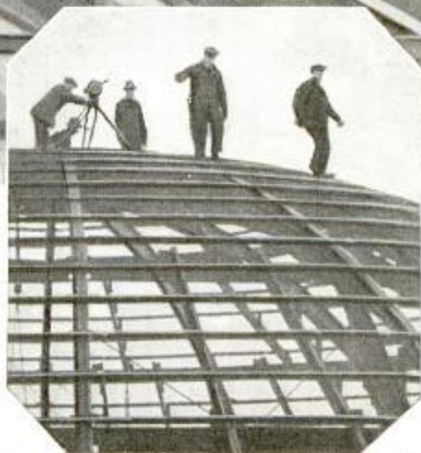
Photographer Climbing Unfinished Building to Get Picture from the Dome, Shown in Insert
