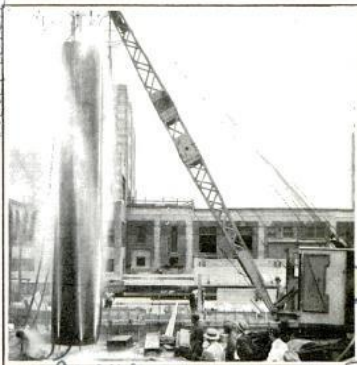
Photo, Frank M. Hallenbeck Giant Caisson Tube Digging Its Own Pit by Means of Water Jets on a Big Bridge Project in Chicago
