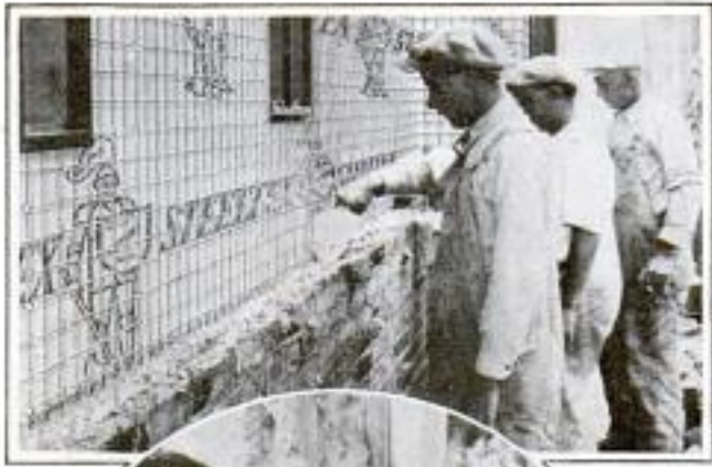
Grouting Mortar to Fill Wall Space, Left; Applying Insulation, Below, and Sketch of the Interior and Exterior Construction of the Wall
