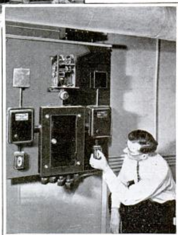
Top, One of Cool-Air Wall Vents; Center, House That Was Cooled; Below, Control Panel
