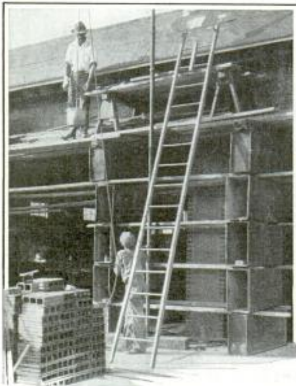
Scaffolding Supported by Discarded Ice Tanks Is Quickly Torn Down without Damage to Material
