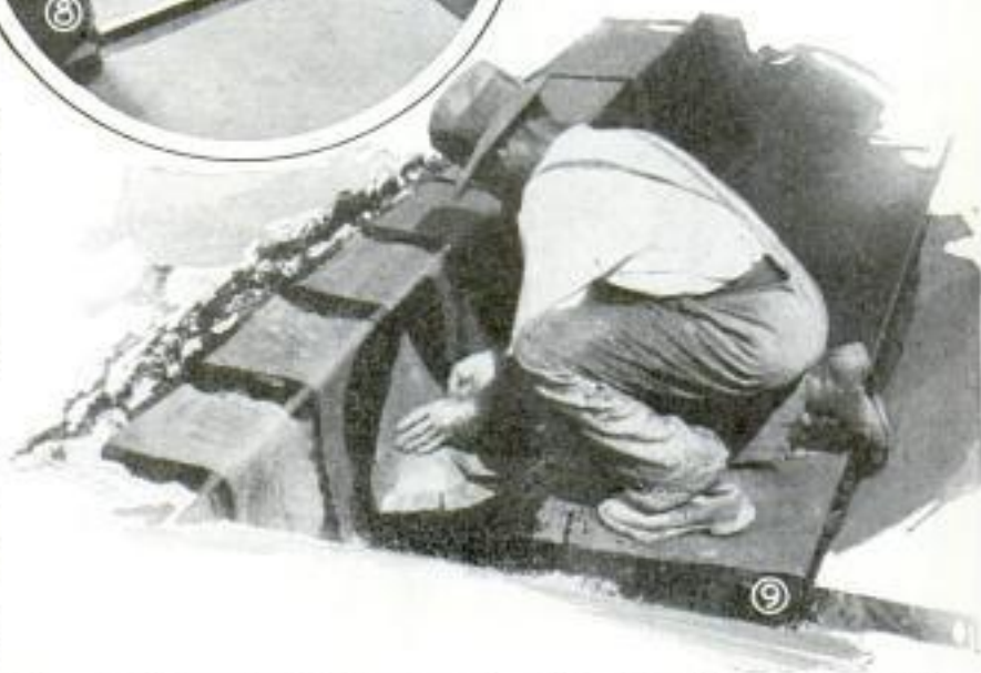
Top and Center, Applying Weatherstrip to Keep Out Draft; Bottom, Workman Repairing Roof before Insulating the Second-Floor Ceiling
