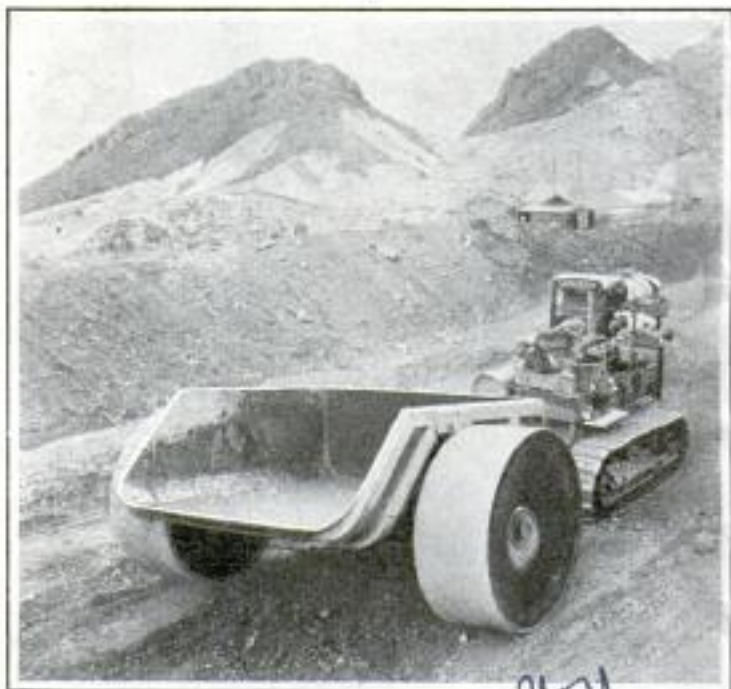
One of the "Roman Chariots" Used in Making a Road to Hoover Dam; the Wide Wheels Prevent Tipping
