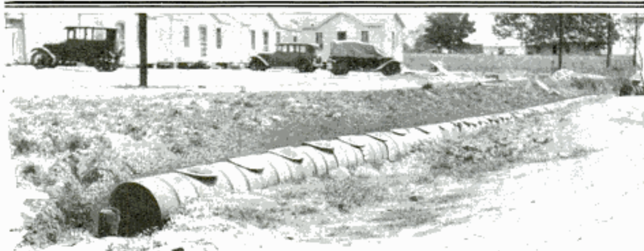
Discarded Oil Drums with the Ends Removed Were Used by a Tourist-Camp Owner to Make a Culvert over the Grader Ditch between His Camp and the Highway
