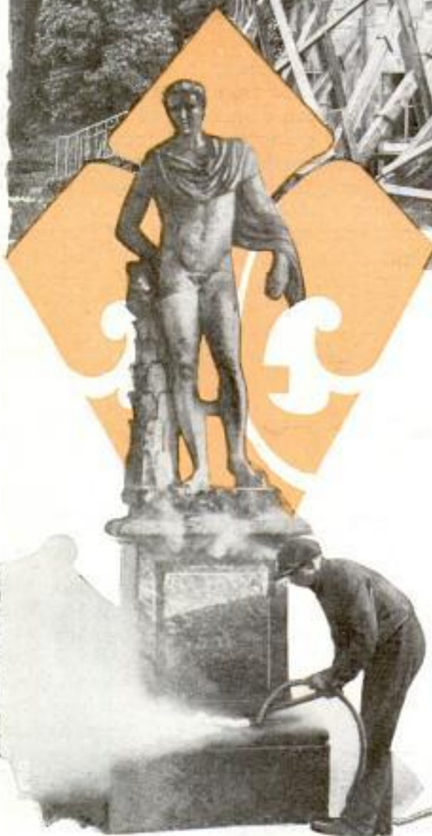
House in Marie-Antoinette's Playground Being Repaired; Below, Cleaning Statues by Steam Process
