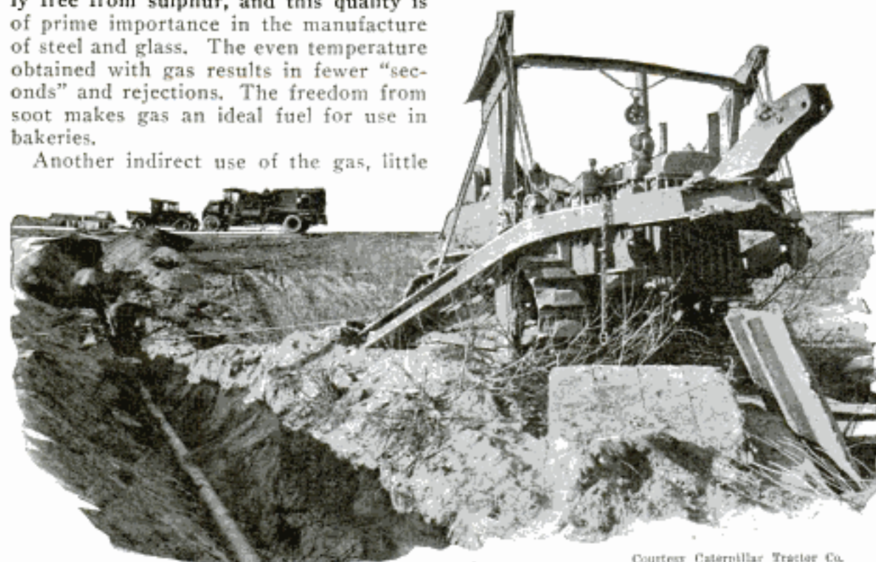
Three Sections of Eight-Inch Gas Pipe Are Laid through Hills and Mountains near Fresno, Calif.; Wherever Possible, the Trenches Are Dug by Tractors
