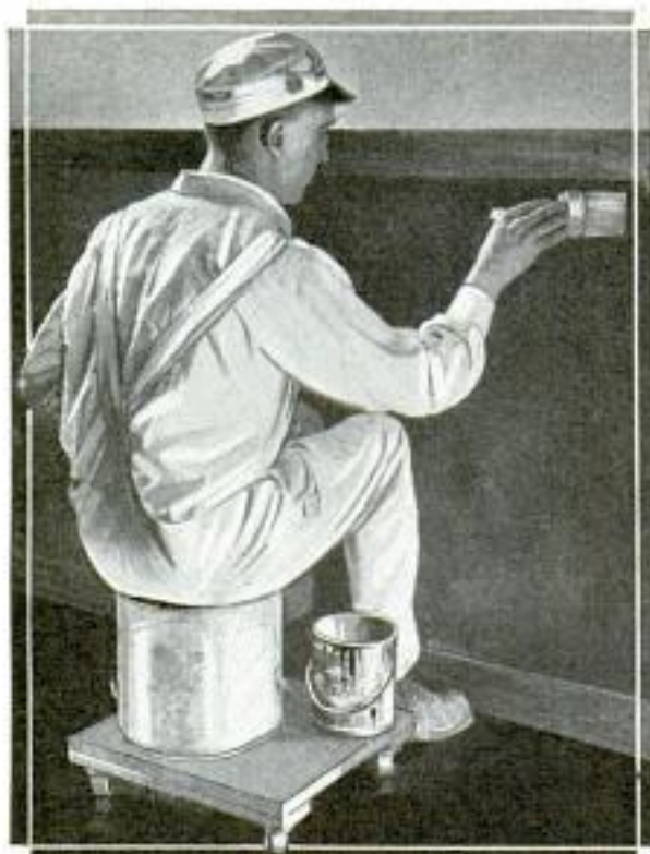
Low Platform Fitted with Casters Provides a Seat for the Painter in Wainscoting Walls
