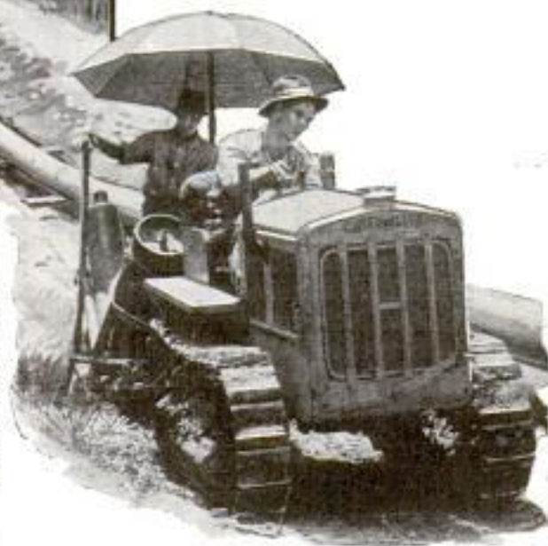
Welding the Joints of a Georgia Pipe Line; a Tractor Hauls the Equipment through the Cane
