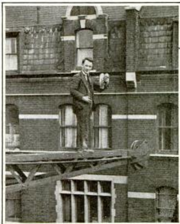
Portable Crane Used to Reach Nesting Places of Pigeons That Damage London Buildings
