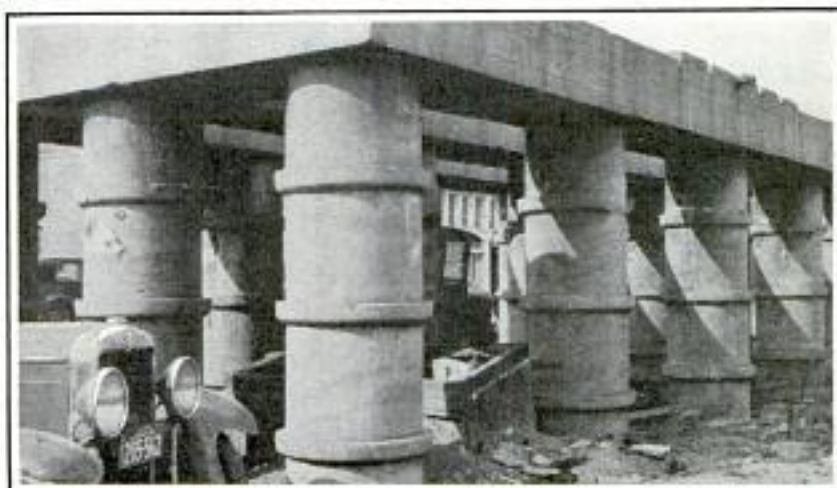
Sections of Large-Size Concrete Sewer Pipe Can Be Quickly Set Up to Provide Durable Forms for Viaduct Pillars
