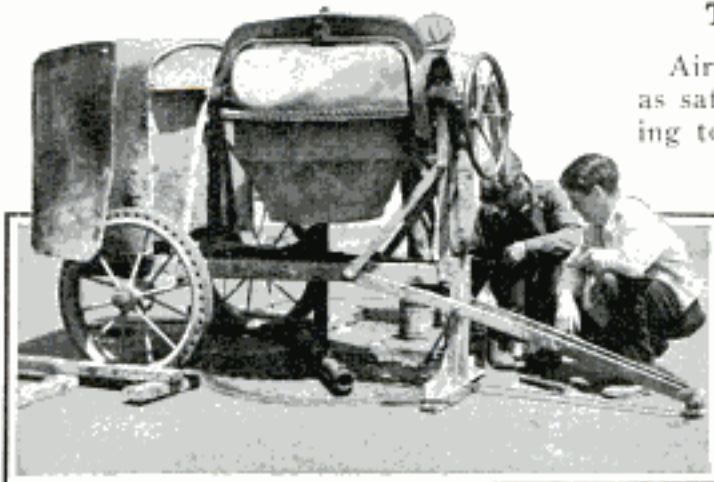
Grinder for Manhole Covers Fits the Lid to Its Seat; Noise from Auto and Truck Wheels Is Reduced
