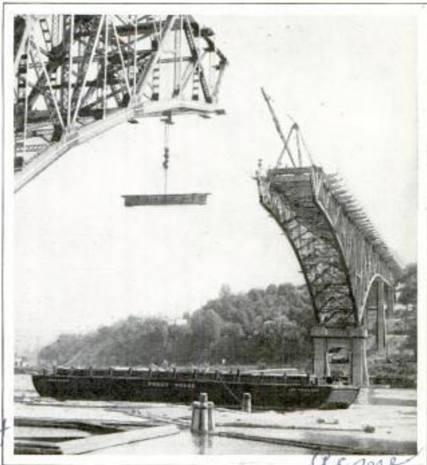
Up and Over; Center Span of Lake Union Bridge at Seattle, Which Is Nearing Completion, Shortening Route into City
