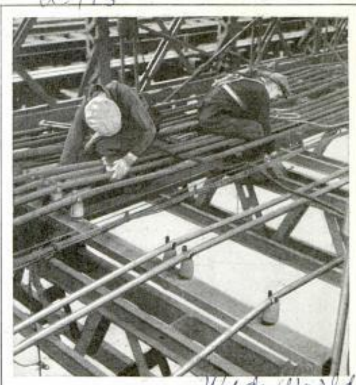
Workmen, Equipped with Life Belts as Protection in Case of a Fall, Removing Power Cables from Brooklyn Bridge
