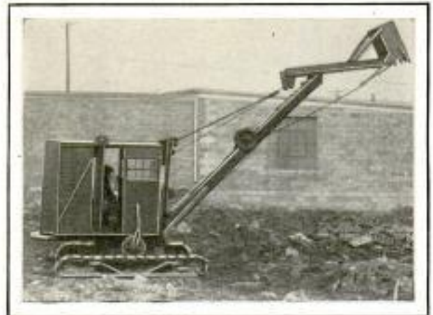
Power Shovel Operated by Gasoline Engine Which Can Handle 10,000 Cubic Yards of Dirt a Day
