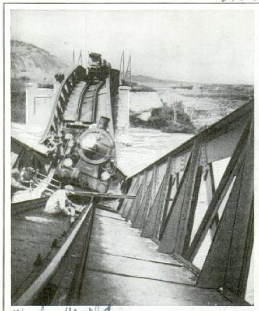
Sagging Railroad Bridge in Sicily Which Collapsed with a Train on It during a Cyclone; No One Was Killed or Even Injured
