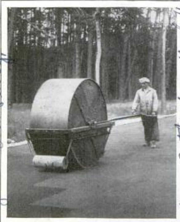
Heavy Road Roller Easily Operated by One Man; It Is Driven by a Motor inside Drum
