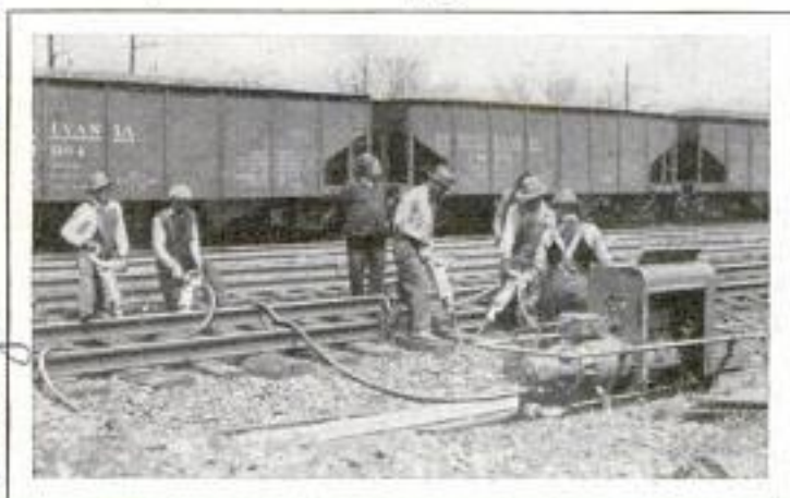
Electric Tie Tamper Operated by a Portable Power Plant: Several Tampers Are Run from One Power Source
