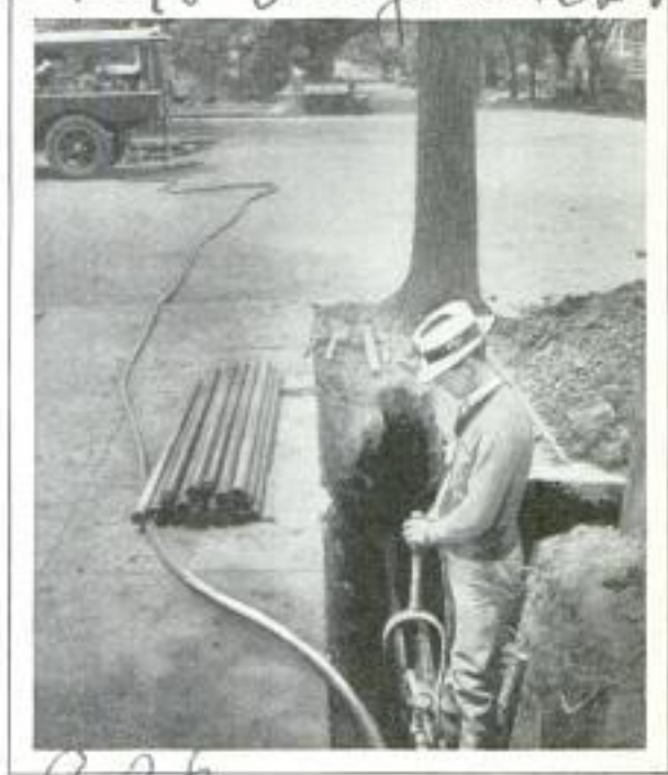
Hydraulic Auger Which Bores Holes for Pipes under Streets without Disturbing Pavement
