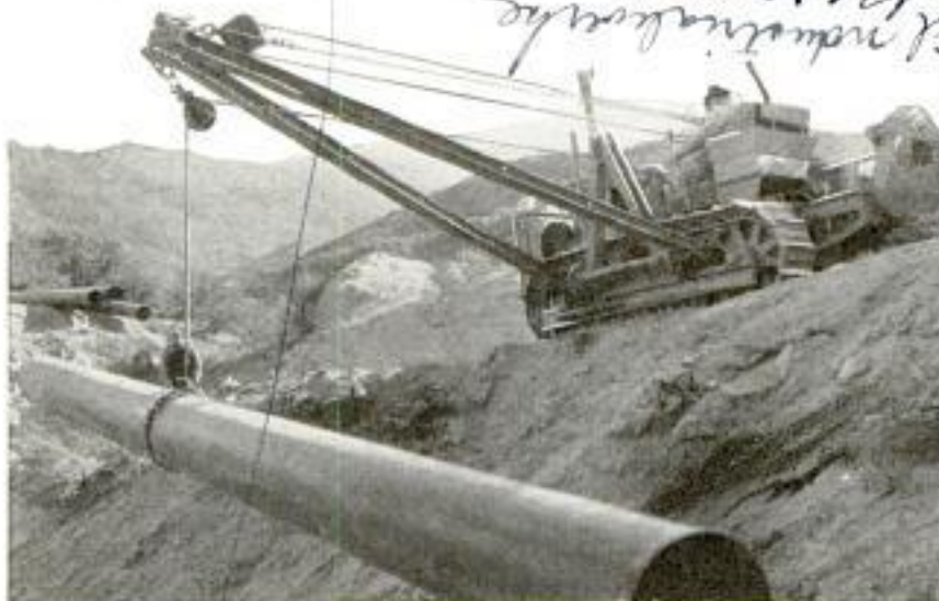
Photo Ewing Galloway Swinging Heavy Length of Gas Main into Ditch with the Tractor Crane Which Saves Hand Labor
