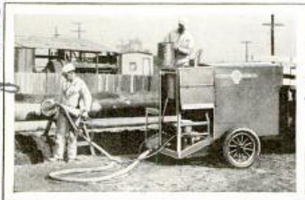
Portable Outfit Used for Coating Pipe Lines with Cement Mortar to Prevent Corrosion
