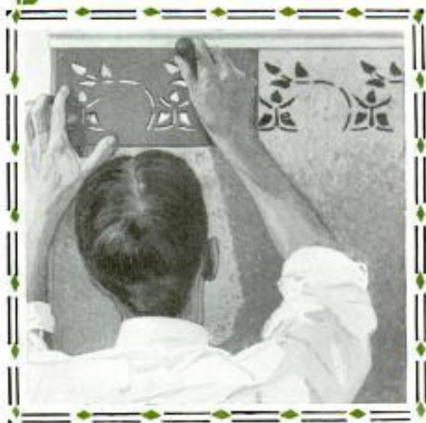
Applying the First Stencil Color of a Two-Part Stencil Border on a Wall
