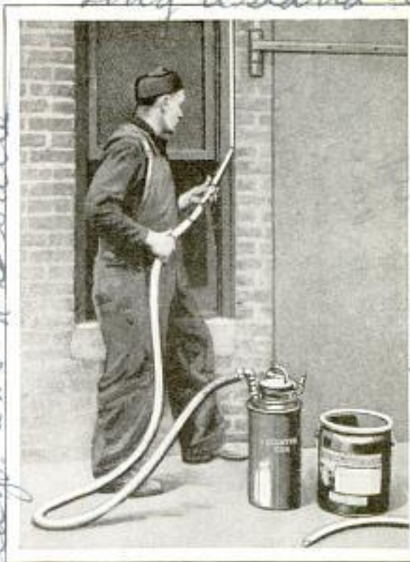
Pressure Gun Being Used for Calking; Usually It Is Operated with Liquid Carbon Dioxide
