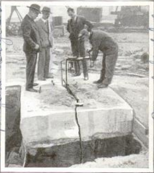
Cracking Large Block of Concrete by Hydraulic Pressure, Thus Eliminating Danger of Explosives
