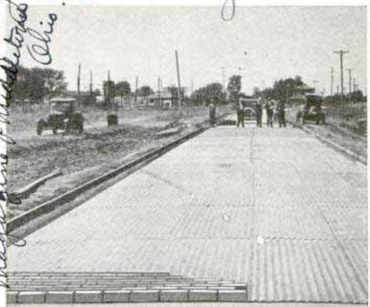
Corrugated-Iron Base for Brick Highway; Sheets of Iron Have Been Found Both Durable and Economical
