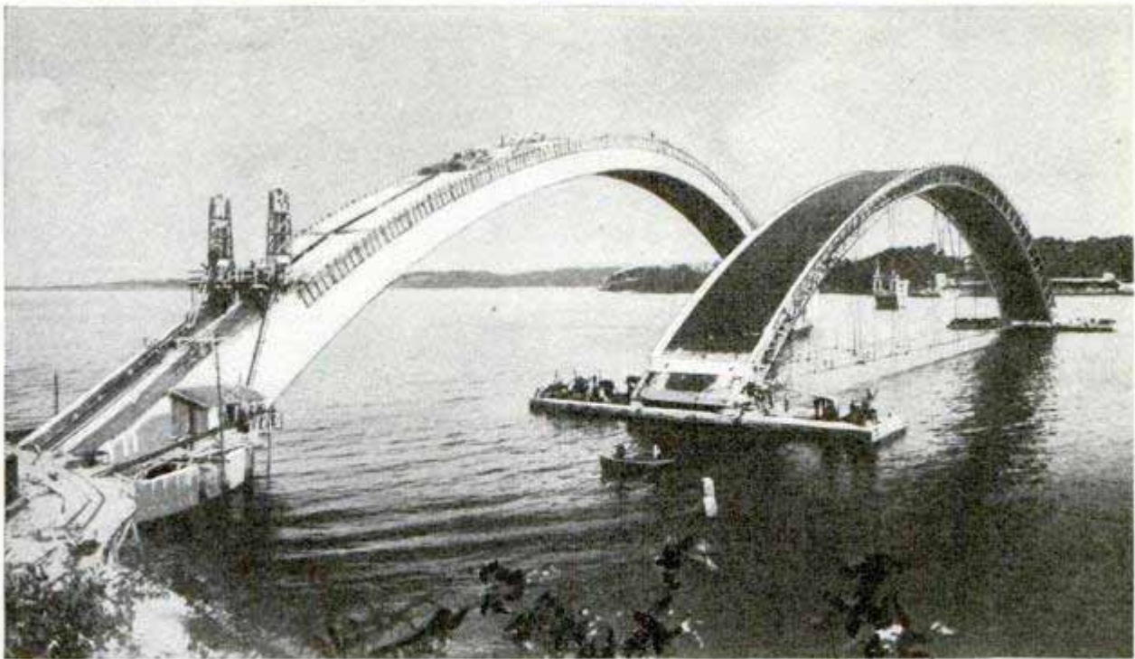
To the Right Is a Form for a 600-Foot Concrete Bridge Arch Being Conveyed into Position on Pontoons; at the Left, One of the Completed Arches of the 2,600-Foot Bridge
