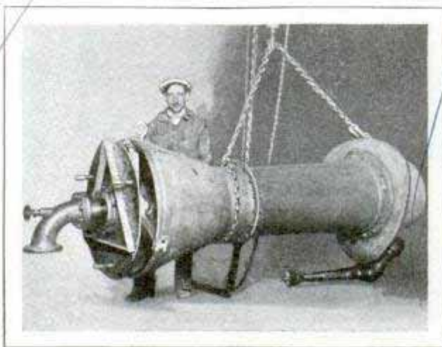
Installing a Huge Gas Burner in a Sugar Refinery; It Consumes 50,000 Cubic Feet an Hour
