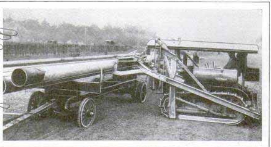
Handling Pipe with the Special Loader-Tractor; the Grappling Arm or Cradle Can Be Lowered for Pushing Dirt
