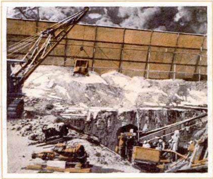
Drilling a Tunnel to a Well to Permit Capping It during a Fire; Several Outlets Were Made below the Surface to Diminish the Force of the Oil and Gas, and So Give an Opportunity for Shutting Down the Well; at Left, beneath This Derrick Is a Well of Record Depth, the Standard Mascot No. 1; It Is 9,629 Feet Deep and Required 458 Days to Drill
