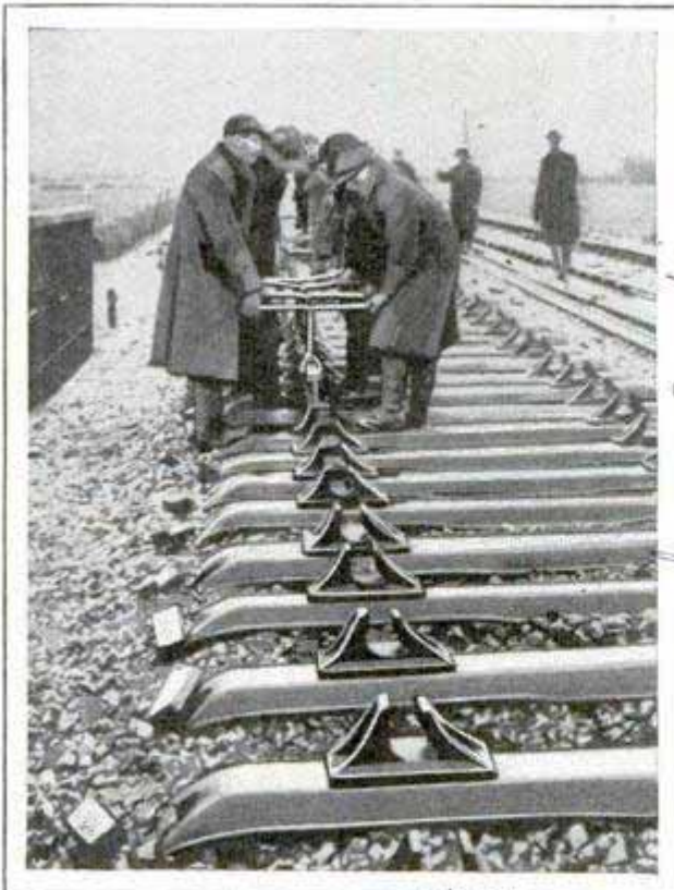
Fitting Rail into "Sleepers" on the Steel Ties Installed on a Stretch of Track in England
