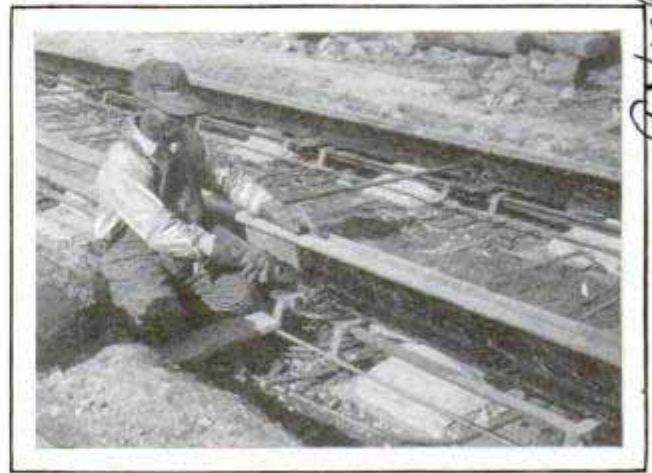
Coating the Sides of Rails of a Noiseless Street-Car Track with Asphalt and Asbestos
