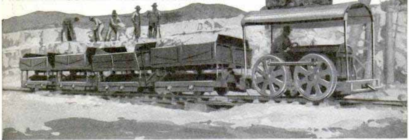
Gasoline Tractor, Equipped with Flanged Wheels to Fit Railroad Track, Serves as Locomotive for Hauling Cars of Dirt and Stone
