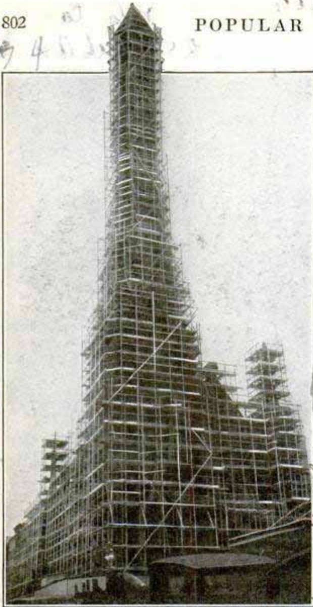
The Steel Frame about This Building under Repair Protects Both Pedestrians and Workmen
