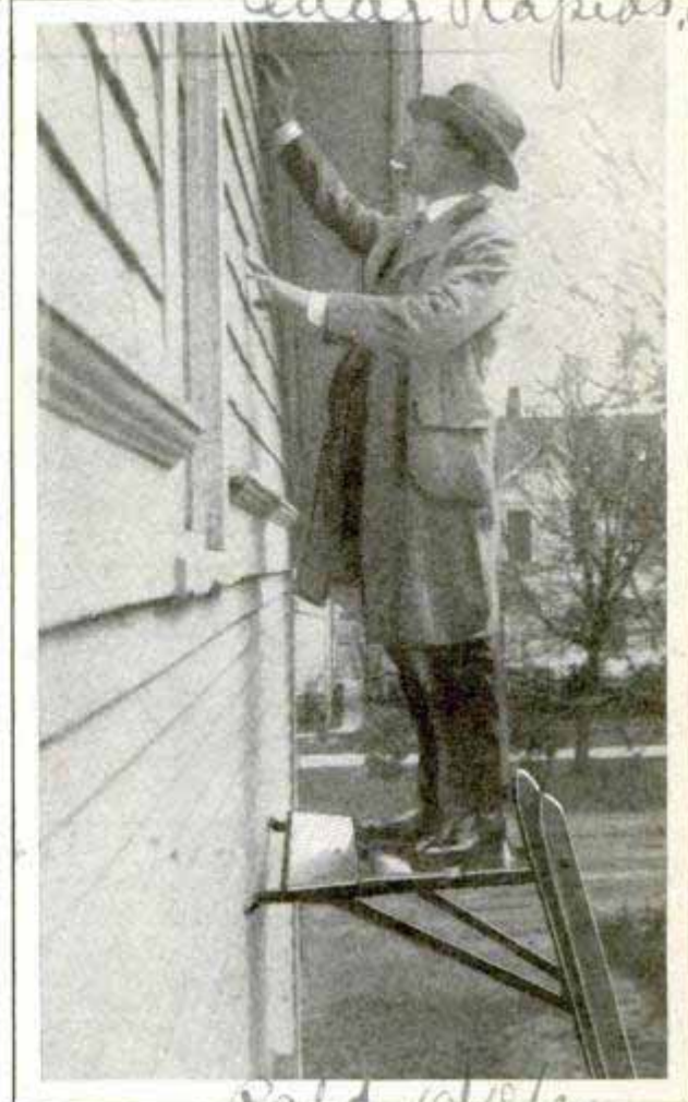
This Platform, Attached to an Ordinary Ladder, Serves as a Scaffold for One-Man Jobs
