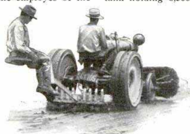
Scraping Excess Tar from Pavements Is Accomplished with This Tractor and Steel-Claw Rake
