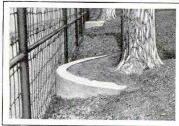
Concrete Curbing, Built around Tree Base on Slope, Retains Moisture, and Adds to the Appearance
