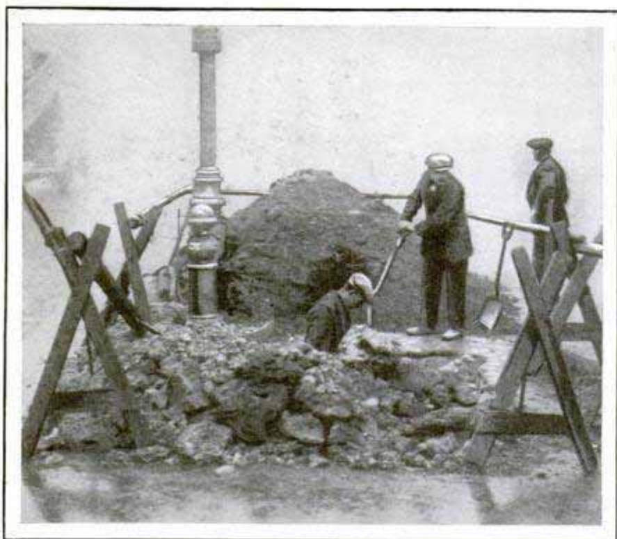
Hunting for a Gas Leak: London Became So Alarmed, Every Smell of Gas Resulted in an Immediate Digging Expedition to Locate the Source
