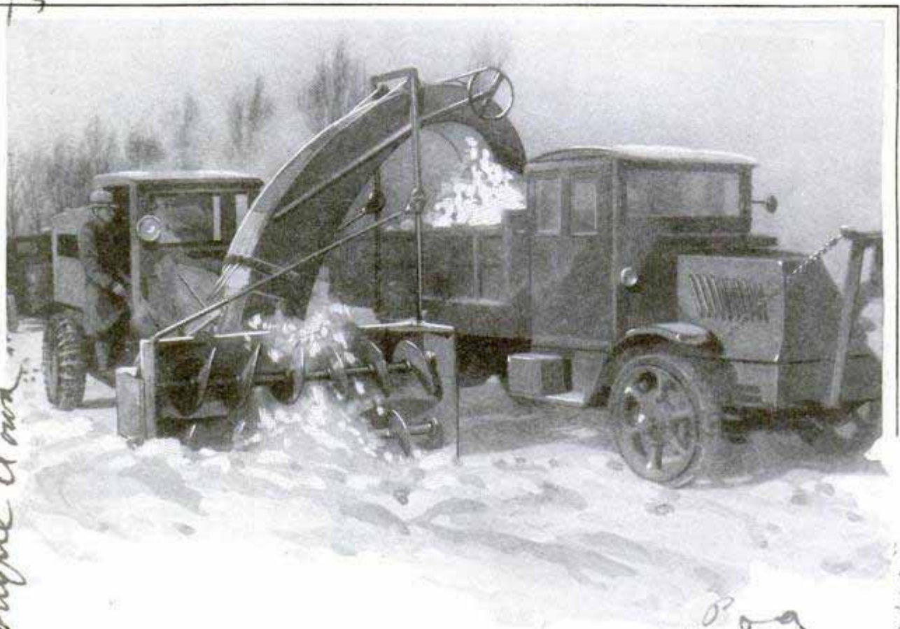
From the Road to the Truck; Removing Snow with the Special Scoop and Conveyor; If the Trucks Are Not Loaded, the Snow Is Thrown to One Side, Out of the Way
