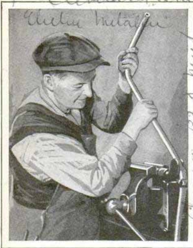
Bending Welded-Steel Conduit for Electric Wiring, Which Eliminates Threading and Corner Boxes
