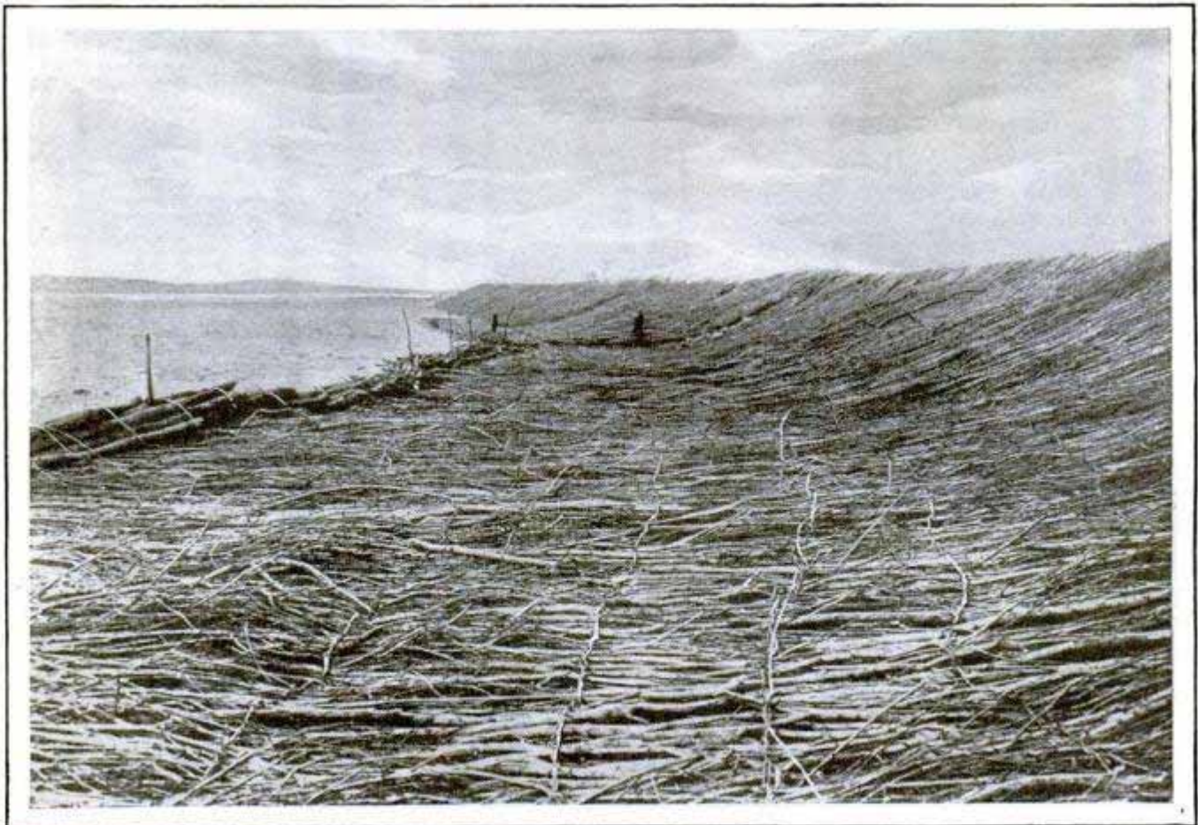
Revetment of Woven Willows Ready for Rock Covering; Protections Such as This Are Spread along Areas Where River Is Weakening Its Own Banks and Those of Levees
