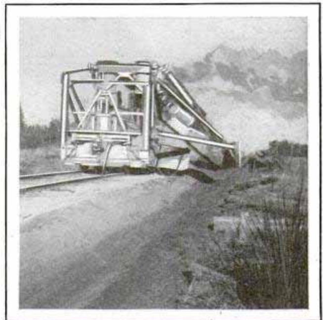
Placing Steel Beams of the Limestone River Bridge; a Sled Load of Duck Boards for the "Front Line," and, at Bottom, a Modern Ditching Machine
