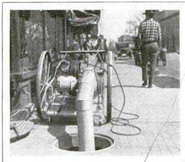
Ventilating Manhole with Pipe and Blower
