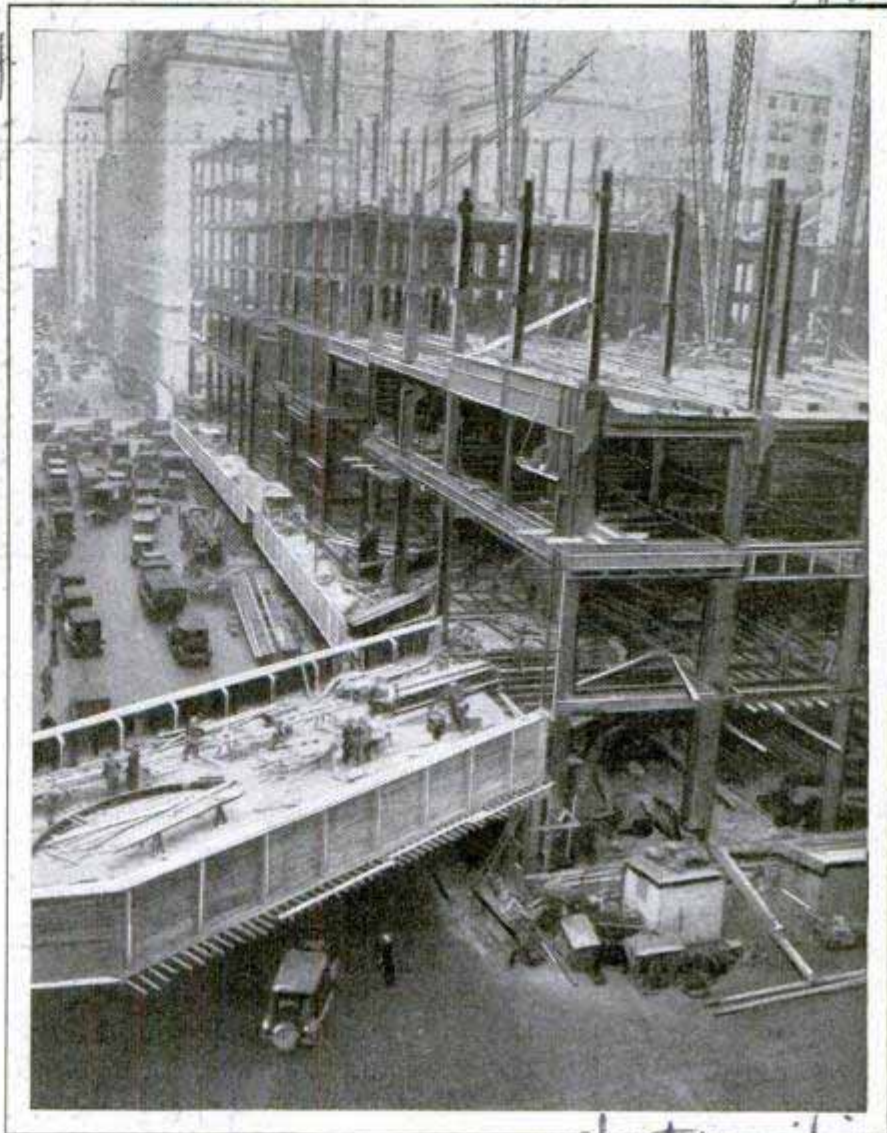
Where Autos Will Pass through a Skyscraper; One of the Drives That Leads into the Huge Building as It Appeared under Construction
