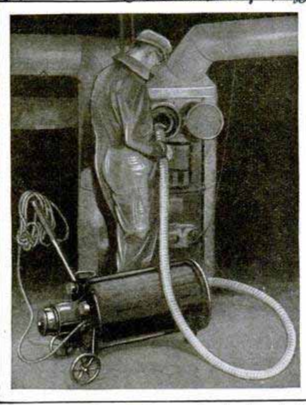
Removing Soot from the Furnace by Suction; Applying Vacuum Cleaner Which Eliminates Dust
