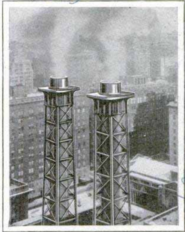
Steel Lattice around High Smokestacks, to Shield Their Unsightly Appearance in Residential District
