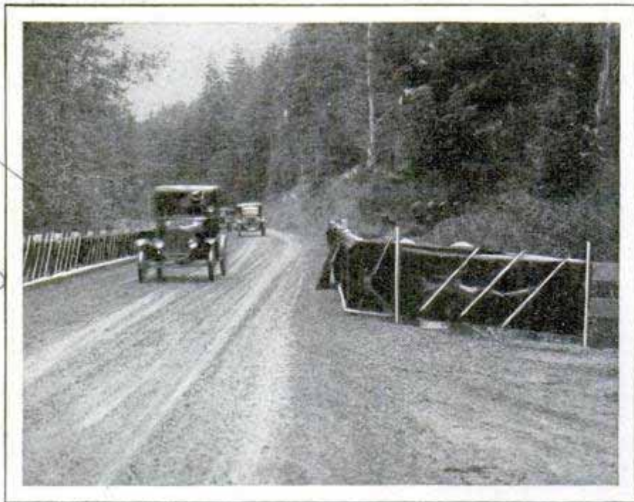
Screen along Roadway, in Oregon, to Prevent Oil from Dripping into the Stream and Killing the Fish
