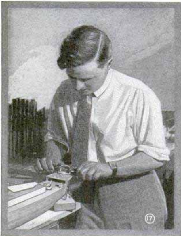
"Crowning" the Surface of the Fo'c'sle Deck; Note Improved Cradle Holding Hull
