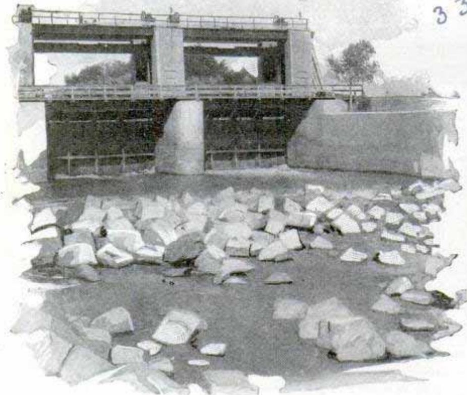
Boulders in Stream Bed to Prevent Water from Tearing Out Bottom and Banks by Breaking Force of Flow
