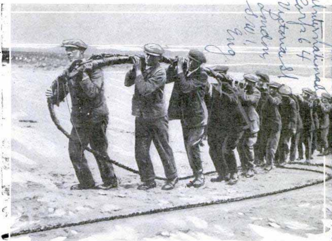
Completing the "Cable Handclasp" between England and Belgium; Placing the Shore End of the Big Line; Special Coverings Have Been Used to Protect the Wires from Corrosion
