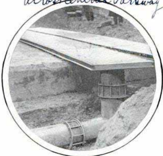
Flat Gas Pipe and Its Connection with the Main Conduit at Point of Crossing under Pavement
