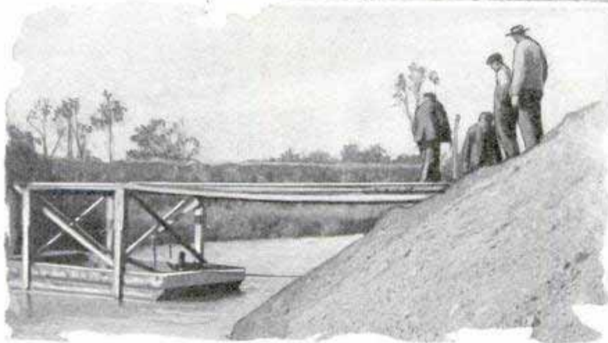
Eliminating the Expense of Building a Trestle for Making an Earth Fill
