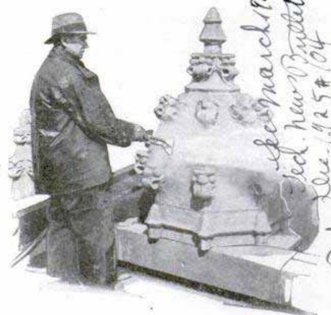
Scouring Building's Decorations with Blast of Steam; an Advantage Is That Crevices Are Cleaned
