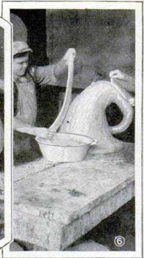
Applying Strips of Burlap or Hemp Soaked in Plaster of Paris, to Add Strength and Thickness to the Wall
