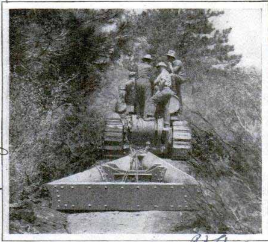
Uprooting and Cutting Brush Likely to Spread Fires; the Plow in Action on California Forest Tract Where Dry-Season Blazes Occur
