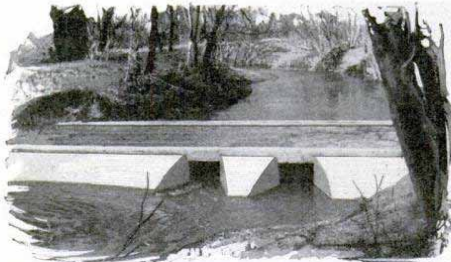
Low Concrete Bridge Permits Flood Water to Run over It, to Prevent Washout, While Normal Flow Passes through Openings
