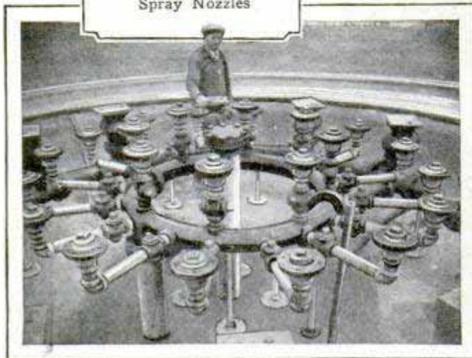
Below, One of the Many Groups of Spray Nozzles
