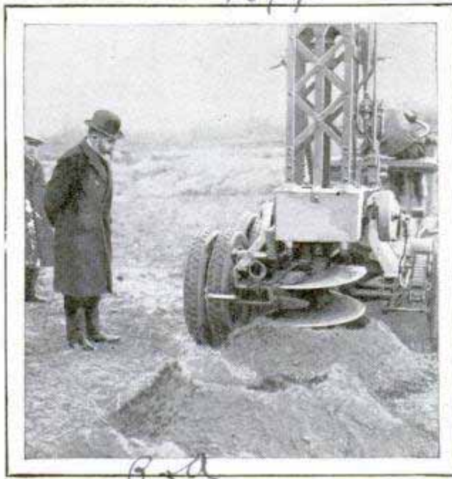
Boring Holes for Trees with the Corkscrew Digger: Dirt Is Piled for Convenient Replacement
