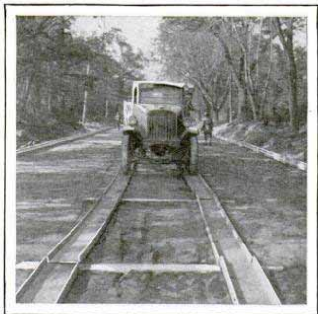
Steel Roadway for Trucks That Protected Subgrade While Pavement Was Being Constructed
