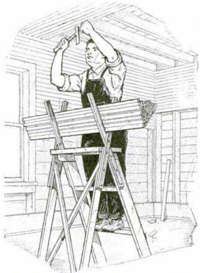
Improved Buck on Top of Stepladder Makes the Work of Lathing Much Easier
