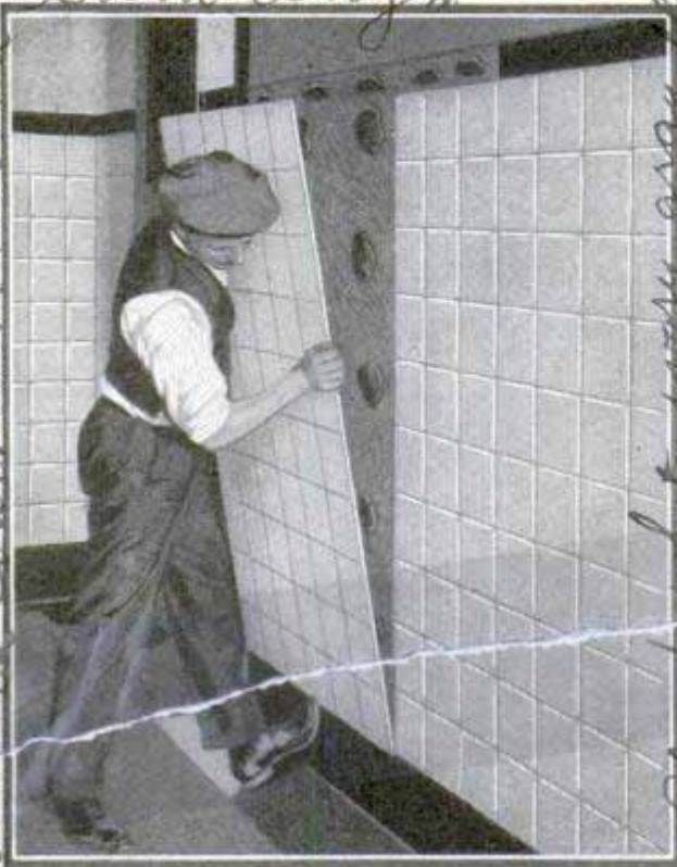
Fitting Slab of the New Tile to a Wall; Its Qualities Permit Using It for Repairs
